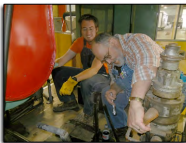
Ethan "Zeke" Dodd and Steve Habeck figuring out the air compressor system on the S.P.L.Co. No.2 logging engine prior to its move from the Art Barn at the fairgrounds.
