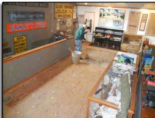
Volunteer Keith Nicoles cleaning up after cutting out the 48-year-old rug from the mezzanine gallery and display space.
