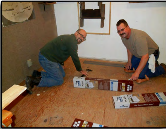
George Schucehenzuber and Marty Swisher begin laying the new flooring in the Mezzanine.
